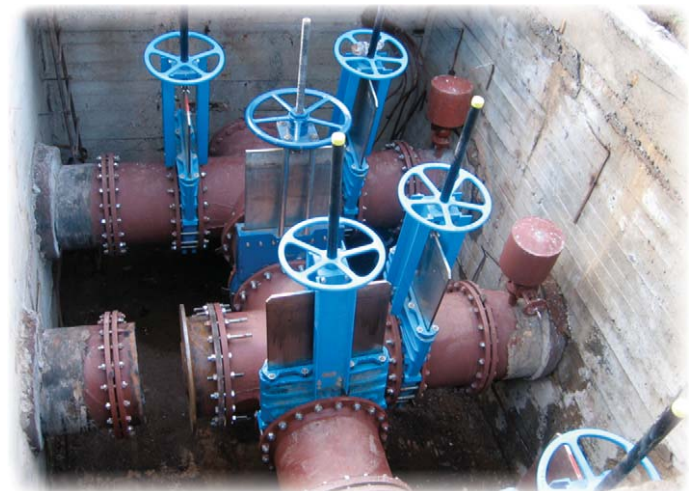
Sewage water treatment application
